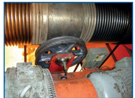
Load Pin SLC installed on an EOT as overload guard.
